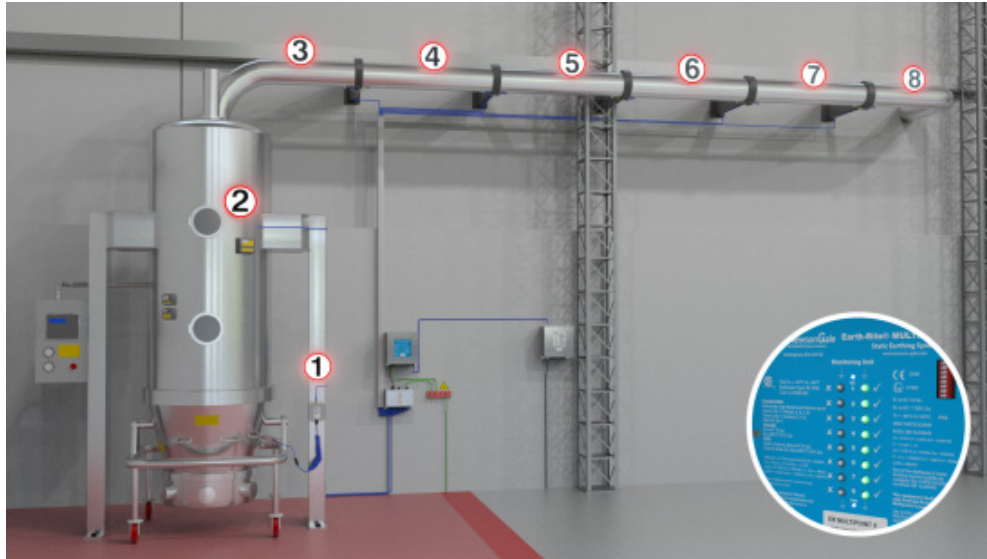
This example demonstrates the Earth-Rite MULTIPOINT II system grounding and monitoring multiple parts of the conveying system which could be at risk of isolation
