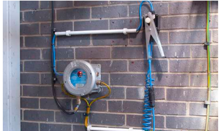
Fig 2. – Newson Gale's mounted Earth-Rite RTR static grounding system. Principally the same as an Earth-Rite MGV, which remains vehicle based
