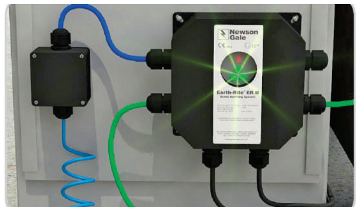
Fig 3. – When the MGV system confirms the vacuum truck is fully grounded, three flashing green high intensity LEDs pulse to indicate that the truck has established a static dissipative ground connection
